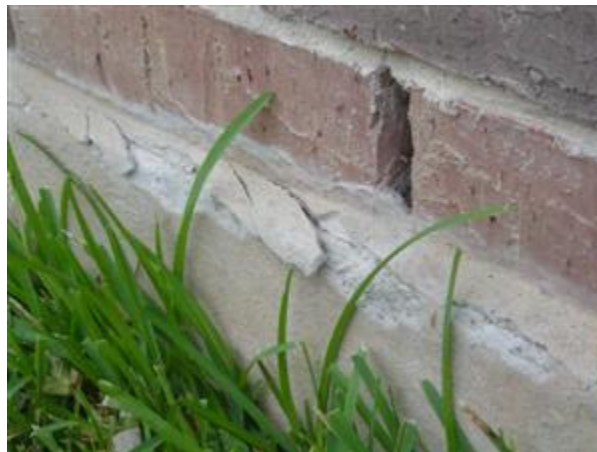
A. Picture 2 More minor cracking
