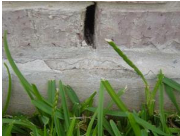
A. Picture 1 Minor Cracking around perimeter
