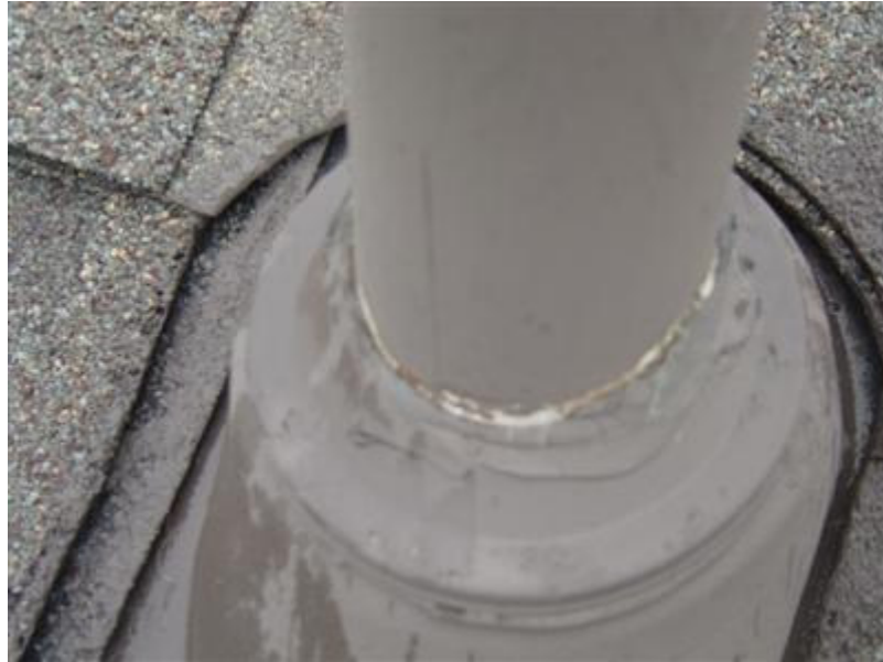
B. Picture 1 Seal broken on plumbing penetration.
