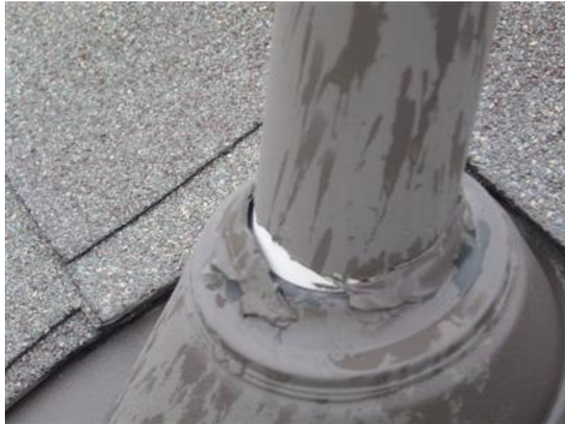
B. Picture 2 Second broken seal
