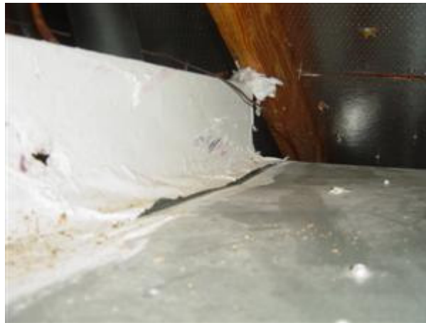
C. Picture 1 Damaged connection - return air connection.
