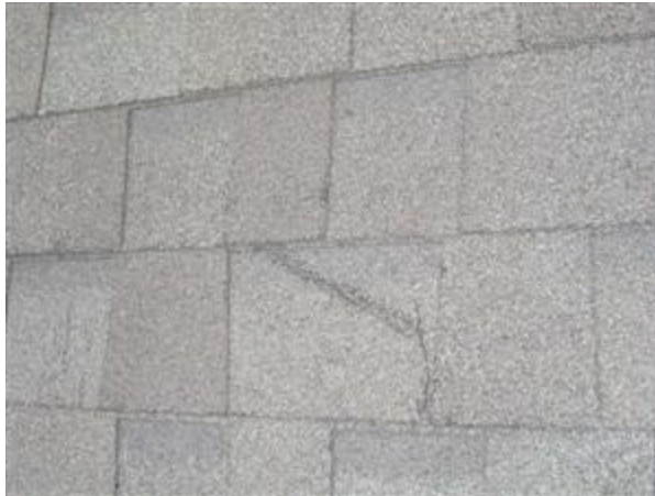
C. Picture 1 Damaged/cracked shingle
